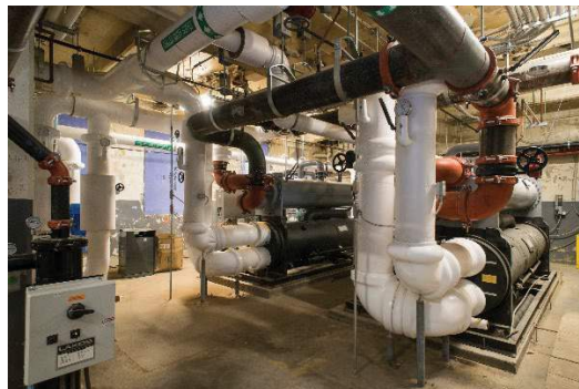
A pair of 375-ton Dunham Bush screw compressors provide supplementary cooling capacity only when economizer cooling is not enough to satisfy the building's cooling load.
