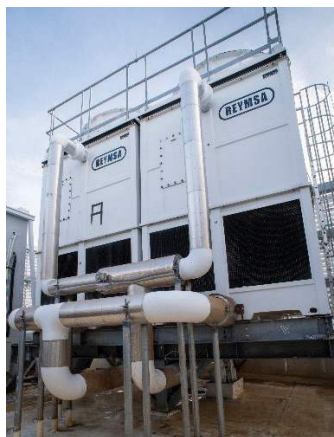
The fiberglass cooling tower used to provide supplementary cooling capacity for The Atlantic's IPS hydronic heating and cooling system.
